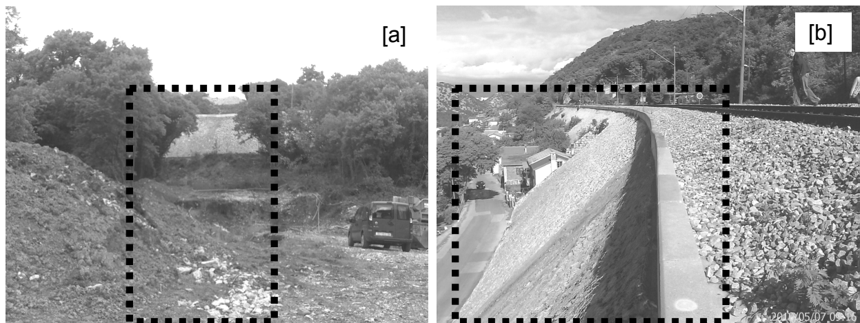
Figure 1. [a] View of the railway embankment from South. [b] Railway embankment with the damage induced by the pipeline HDD installation process before compensation grouting design.
